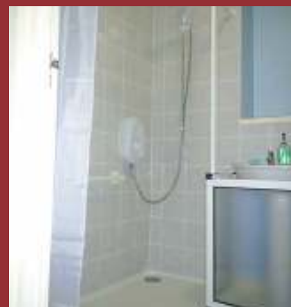
Level entry showers have helped people stay in their home
